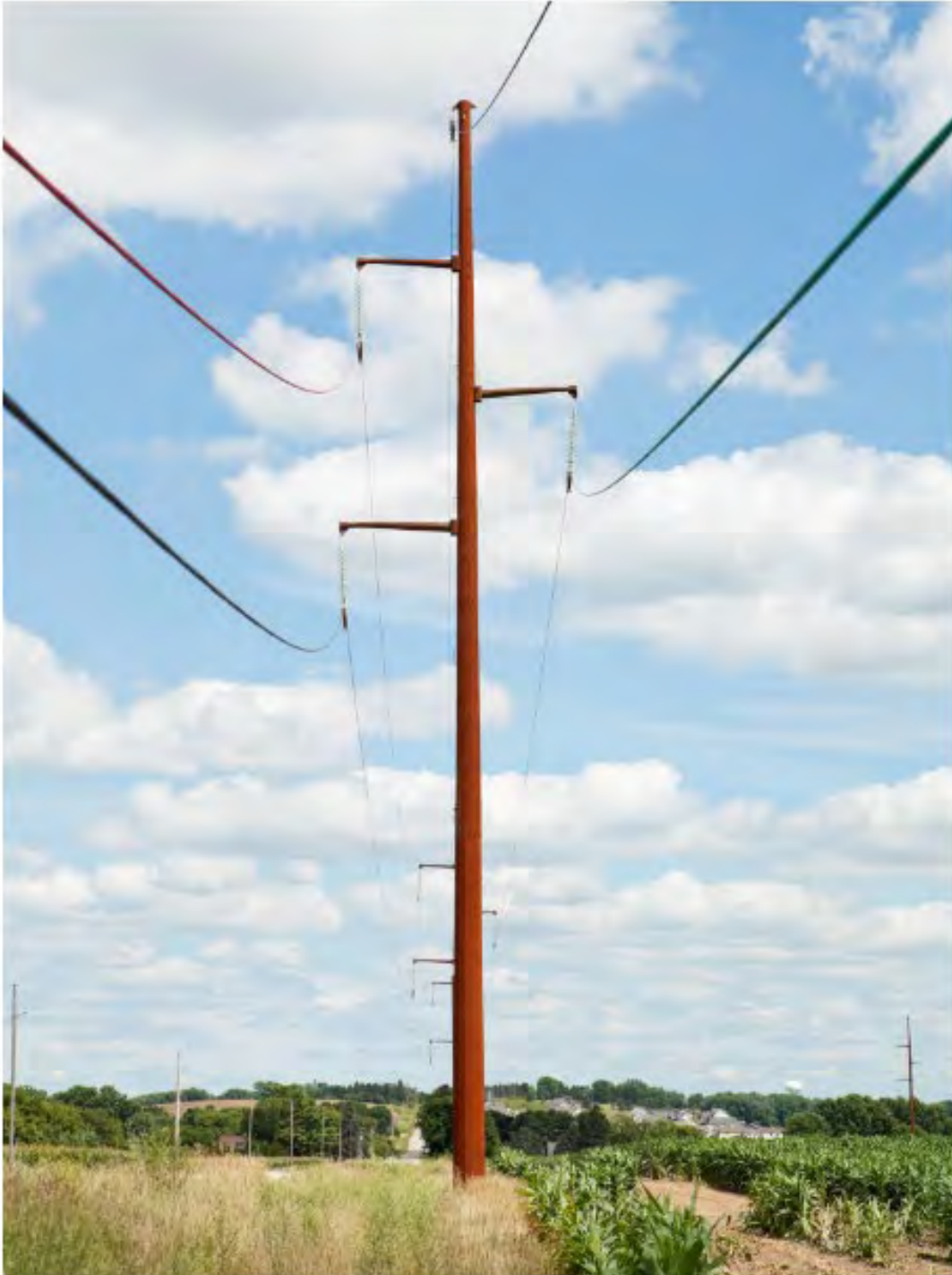
Figure 2-4. Photo of Typical 161-kV Transmission Structure
