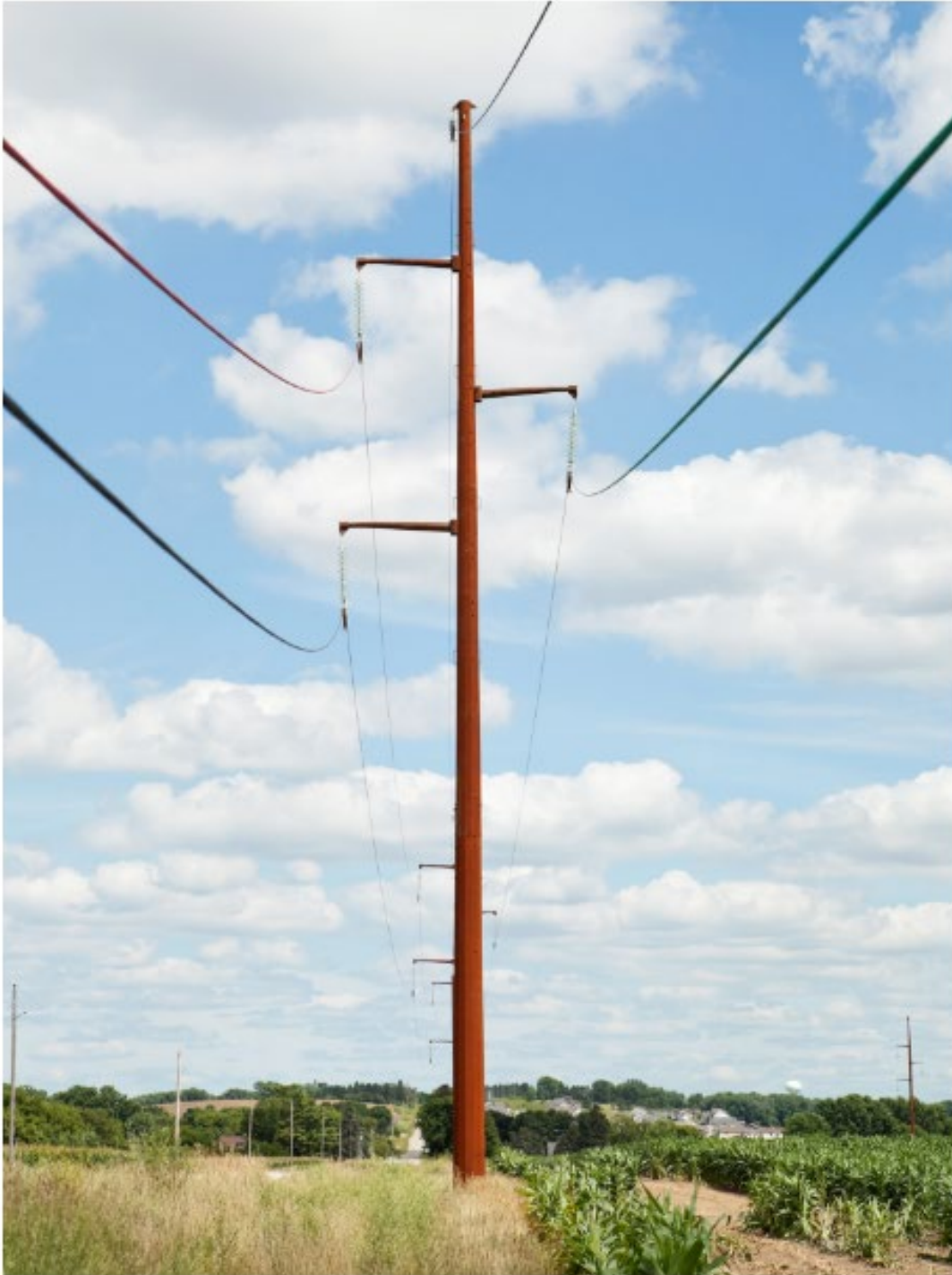
Diagram 3-2. Photo of Typical 161-kV Transmission Structure
